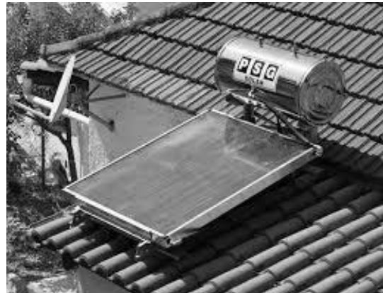
500ltr. Flat plate system in Ranchi Dist.
