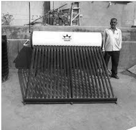
500 ltr. ETC System in Gumla Dist.
