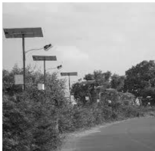
Solar street light in Birsa Jaivik Udyan in Ranchi
