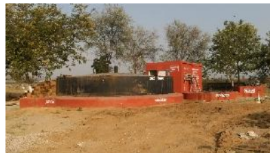
Big bio gas plant to treat 1 ton to 500 tons of waste per day waste
